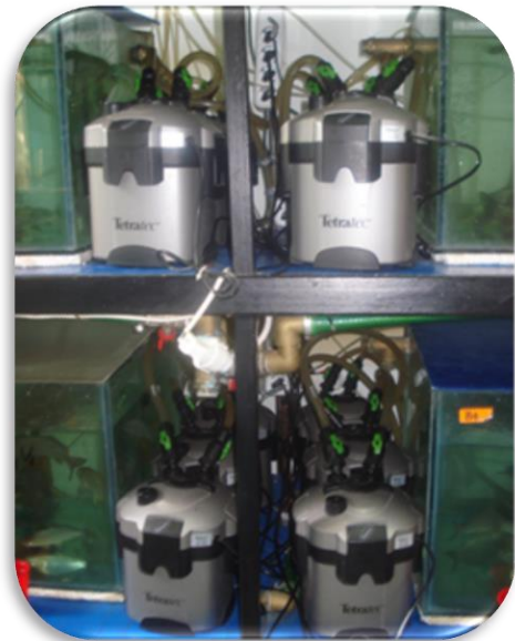
Figure 3. Water quality recirculation and conditioning equipment.
